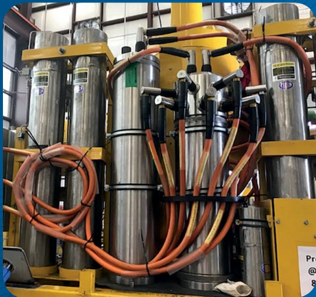
The ODI Nautilus manual mate jumpers shown in the Helix IRS equipment during integration and installation
